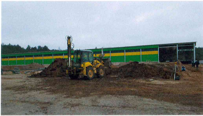
The construction of the incubator (in Lazdijai area); an incubation of about 40 million chicks per year is planned
